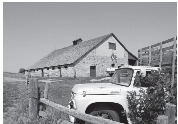
Anderson-Ridley Barn received a Deadwood Fund Grant to assist with repairing mortar and its walls.
