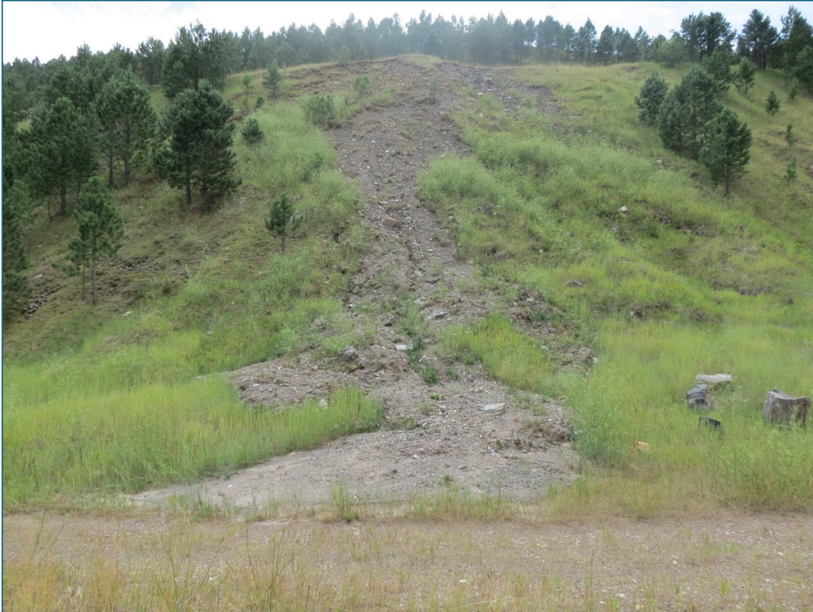
Soil slump in Gayville area prior to 2024 repairs
