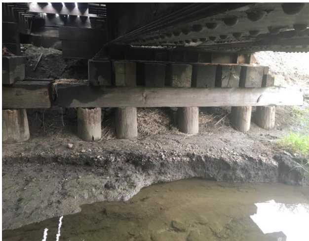
Figure 4: Bridge T512.5 Bent #3 mainline, reflecting hollow pile, remaining poor caps with one missing, splitting caps
