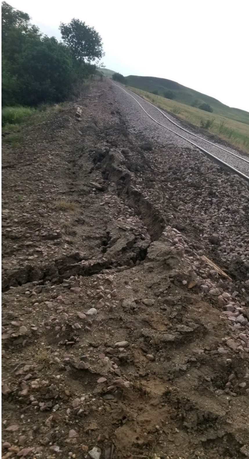
Embankment failure west river
