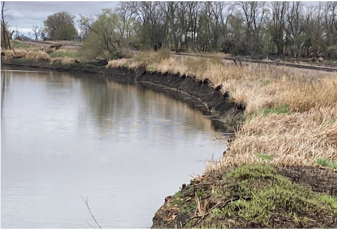
Eroding bank that is moving to within 18 feet of RR ties
