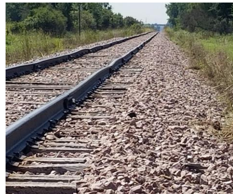
Figure 5: Existing D & I Track Condition with Bent Rail Ends and Rail Warp
