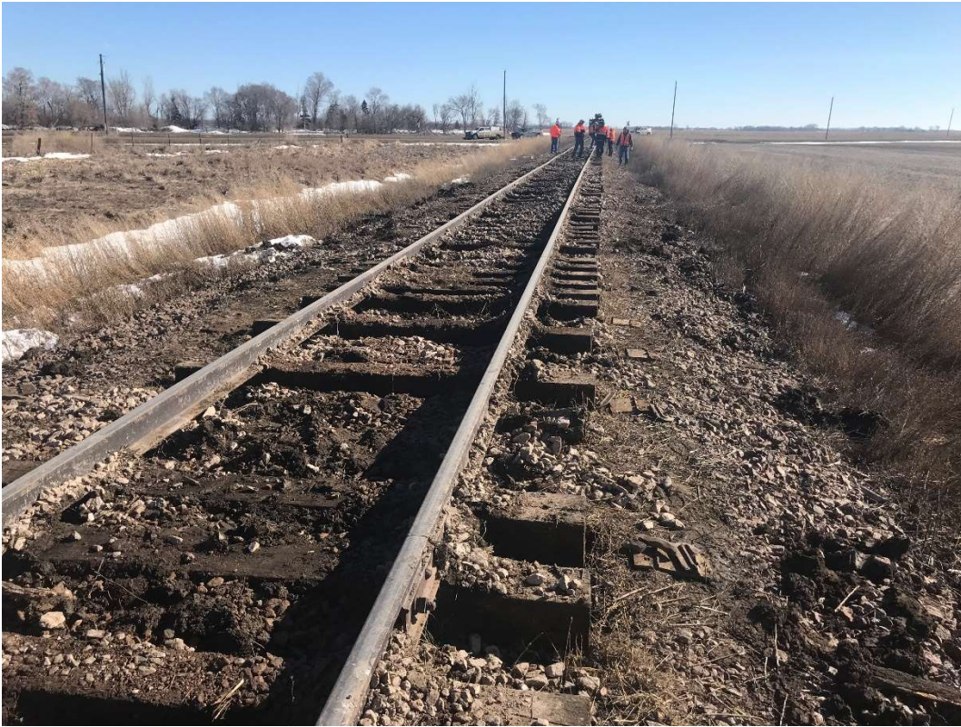
Example of Poor Subgrade and Tie Conditions
