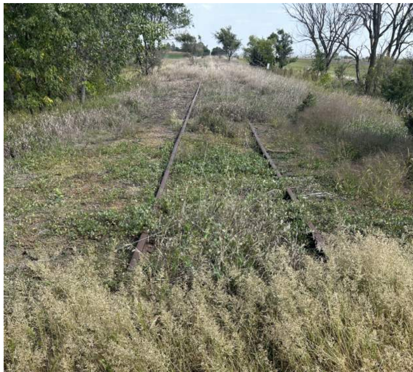
Figures 12 & 13 – General track condition from MP 10.9 to Tyndall (MP 20.9).
