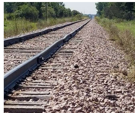
Figure 5: Existing D & I Track Condition with Bent Rail Ends and Rail Warp
