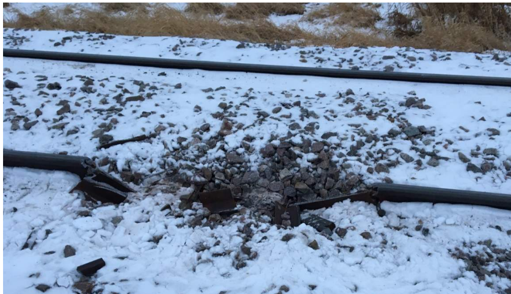
Figures 4 & 5 – Damage to SMRR track caused by derailments.
