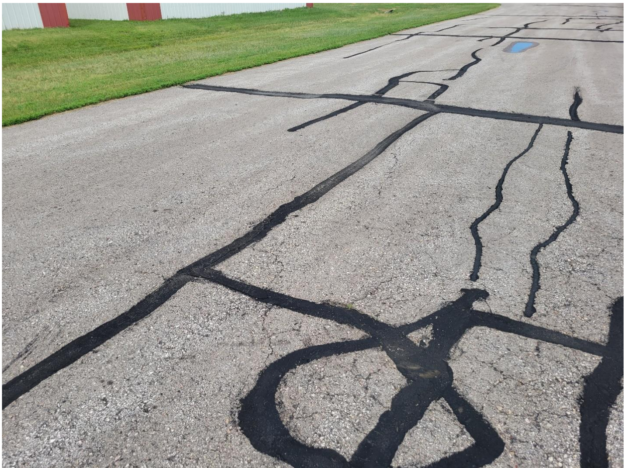
Exhibit 1 - Taxilane after pavement maintenance. Pavement alligator cracked.
