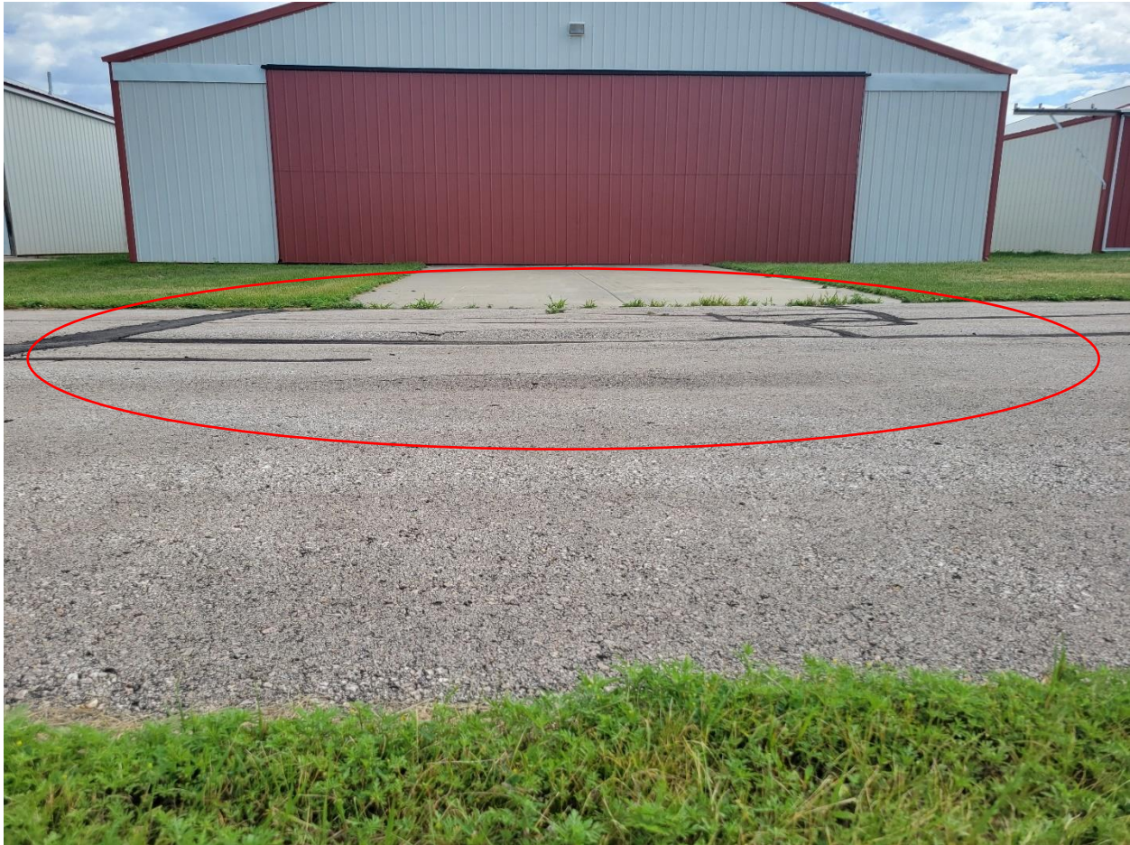
Exhibit 6 - Depression / rut in front of hangar.
