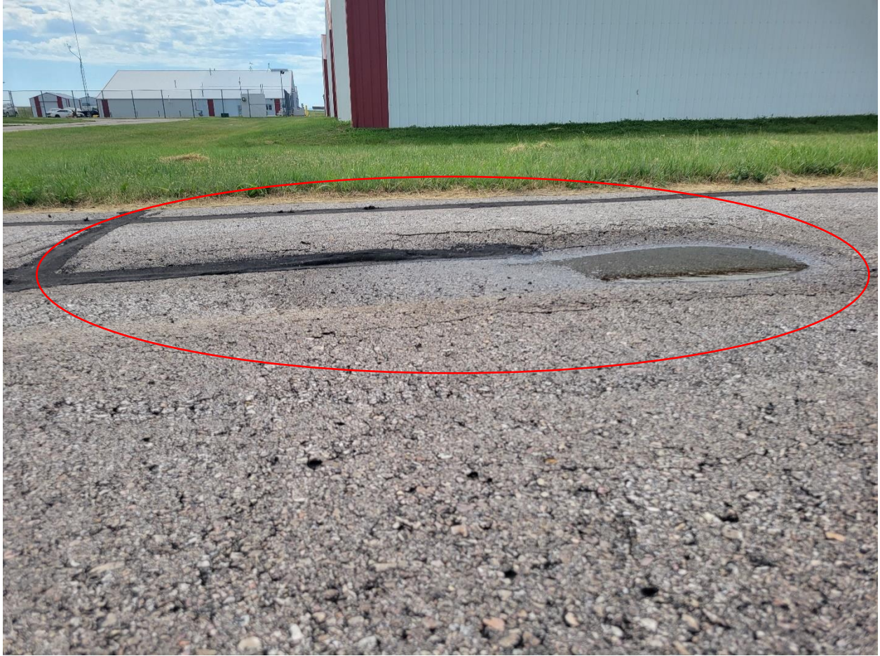
Exhibit 4 - Depression / rut in surface.
