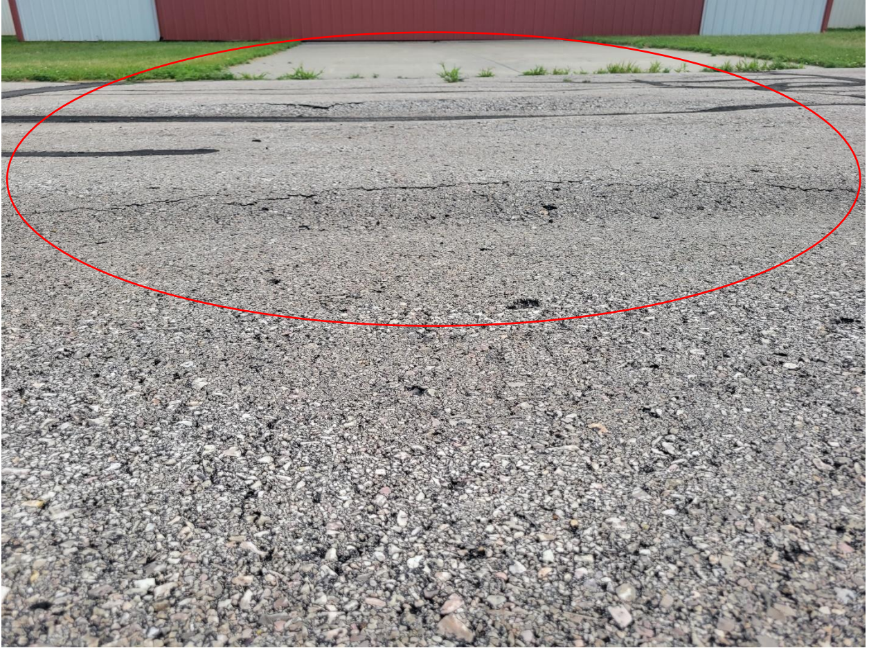
Exhibit 5 - Depression / rut in surface.
