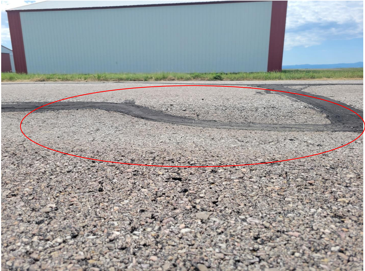
Exhibit 3 - Depression / rut in surface.
