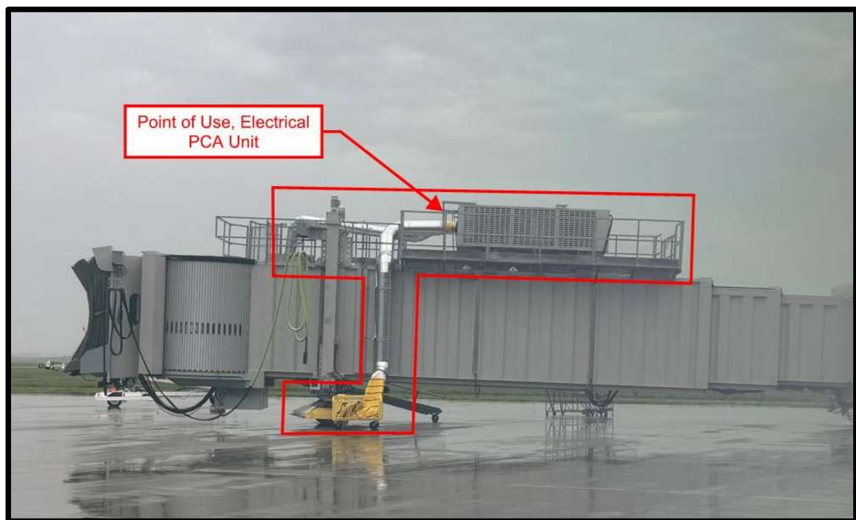
Figure 1: Example of PCA Unit to be Installed
