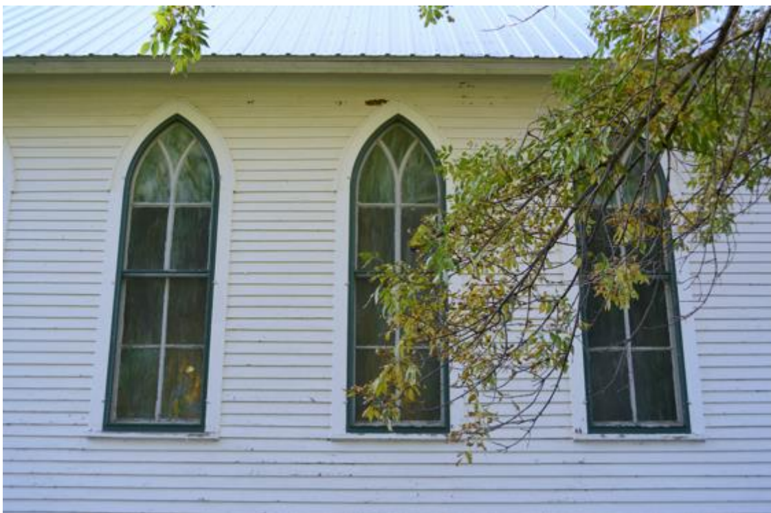
SD_Jerauld County_ Zion Emmanuel Lutheran_0005 Detail of windows on north elevation, camera facing south.
