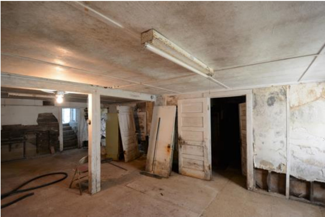
SD_Jerauld County_ Zion Emmanuel Lutheran_0014 Interior view of basement, camera facing northeast.
