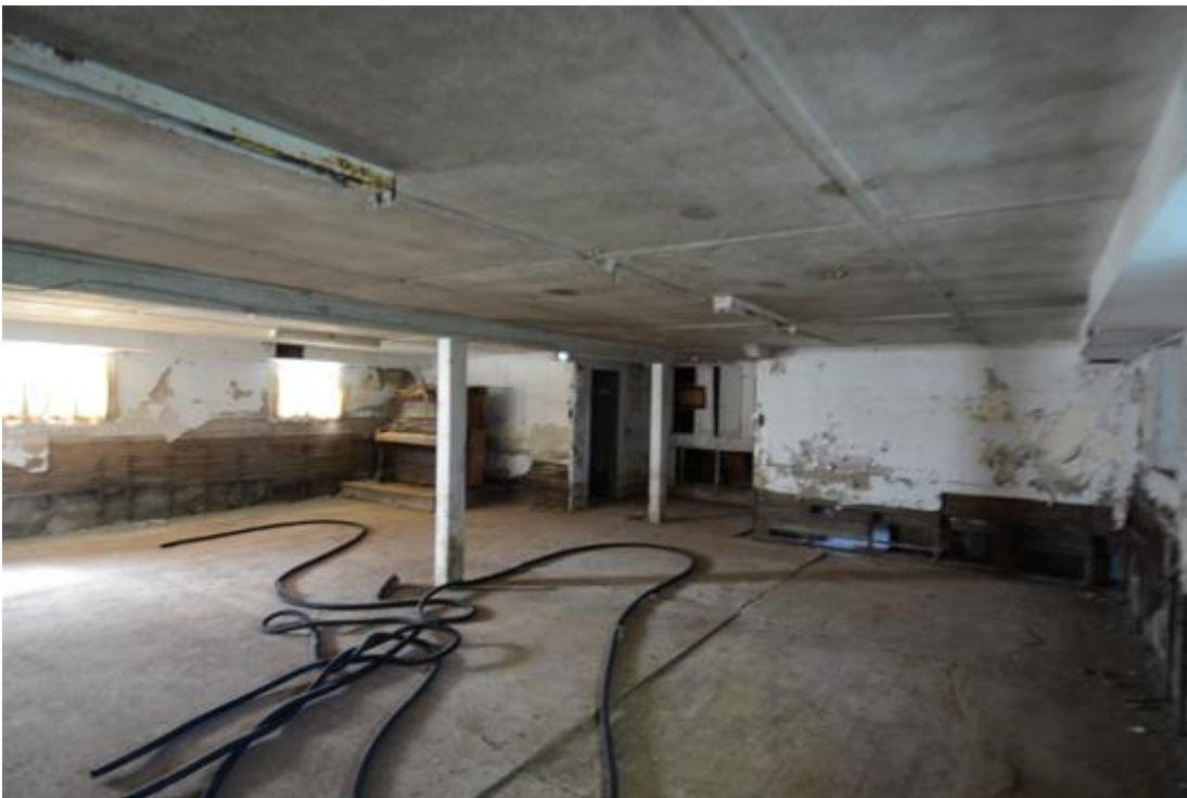
SD_Jerauld County_ Zion Emmanuel Lutheran_0015 Interior view of basement, camera facing southwest.
