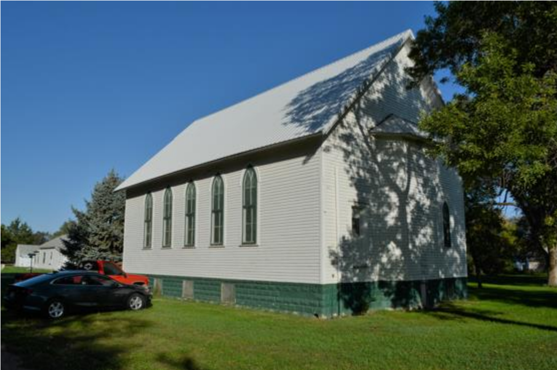
SD_Jerauld County_ Zion Emmanuel Lutheran_0002 Exterior of south and east elevations, camera facing northwest.
