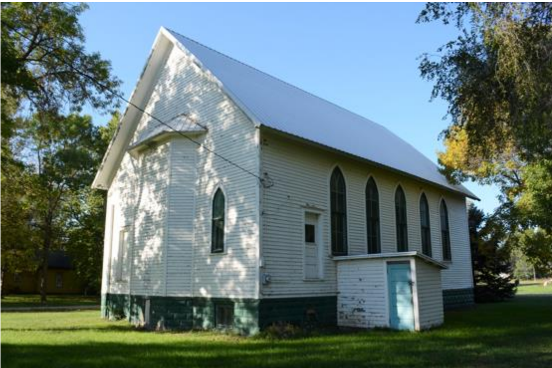
SD_Jerauld County_ Zion Emmanuel Lutheran_0003 Exterior of east and north elevations, camera facing southwest.
